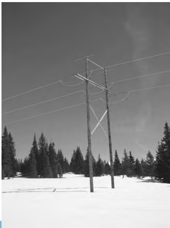
FIGURE 19.1 220 kV line with H-frame wooden towers.
